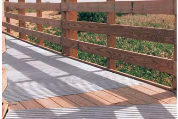
Safe-T-Span pultruded pedestrian grating was chosen for this walkway bridge for swimmers at South Cape Beach State Park near the Cape Cod region of Massachusetts.
