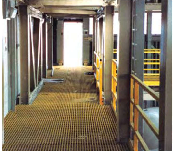
Safe-T-Span pultruded industrial grating at a pulp and paper loading area.
